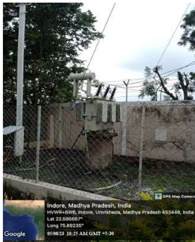
Figure 2.1:- 200 kVA Transformer in the campus
