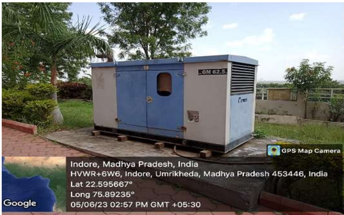
Figure 2.3:- DG set in the campus
