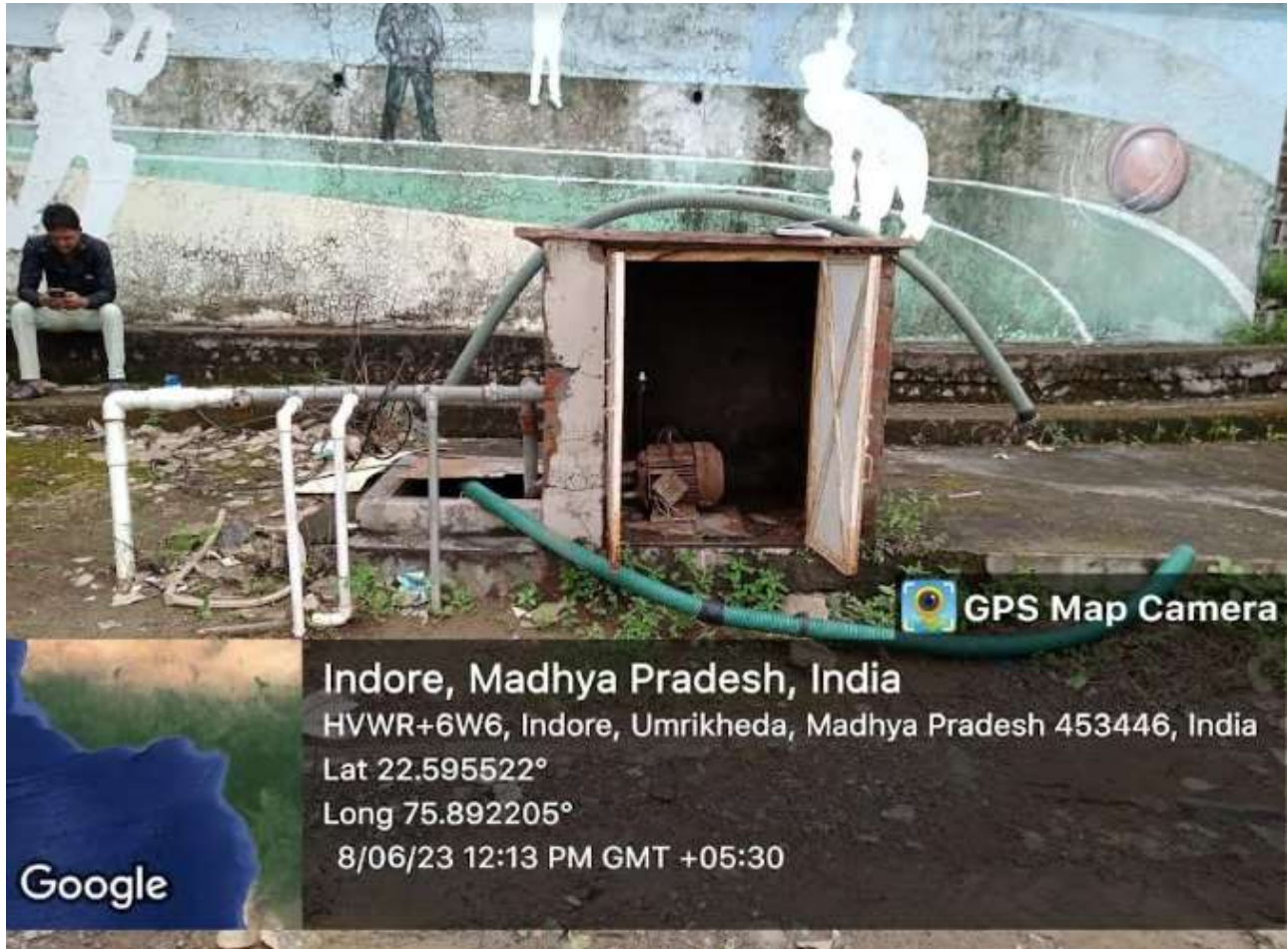
Fig. 2.2 Fresh water pumping station
