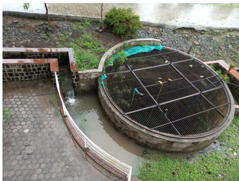
Photograph of Rain Water Harvesting Well
